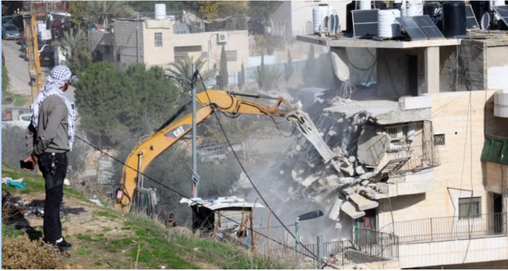
B'Tselem, Israel demolishes a four-story building in Wadi-Qadum, East Jerusalem
